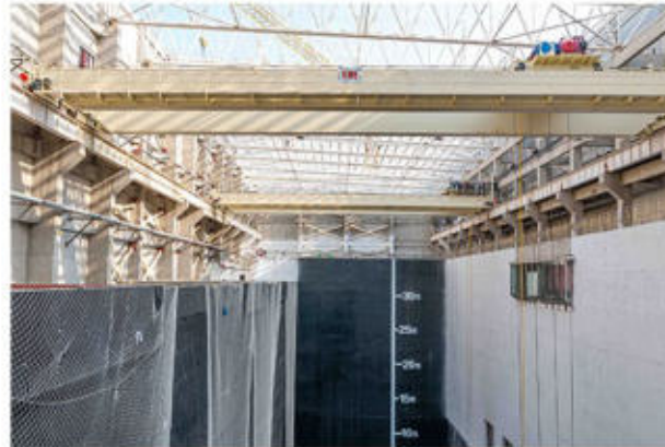
QZ GRAB OVERHEAD CRANE
