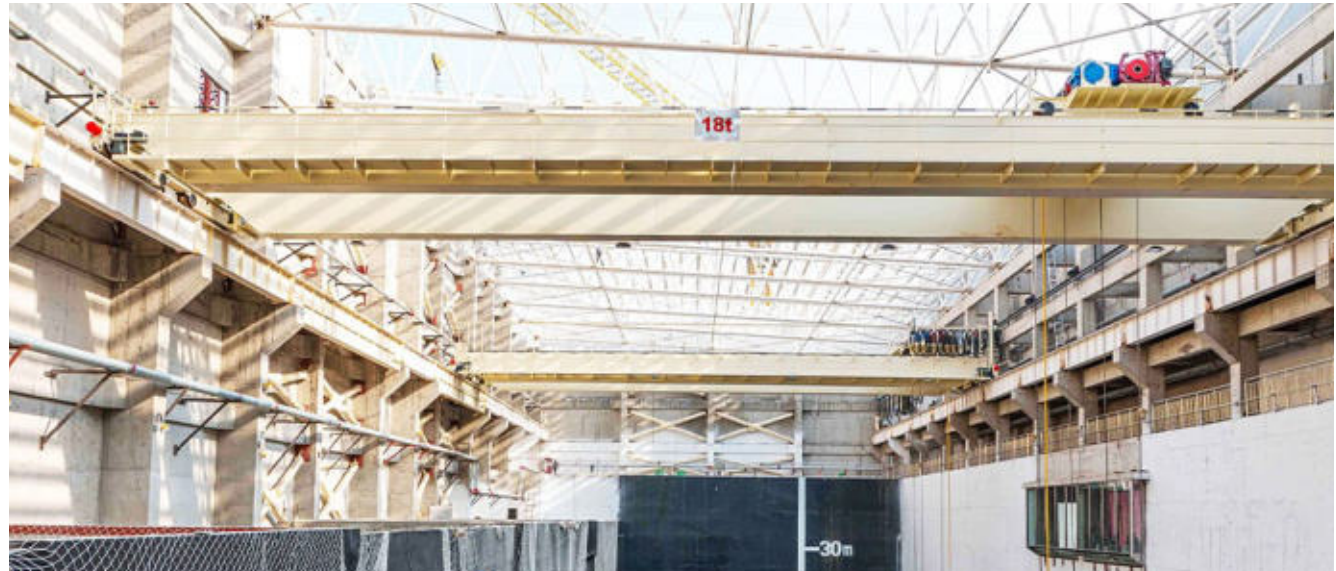
QZ GRAB OVERHEAD CRANE
